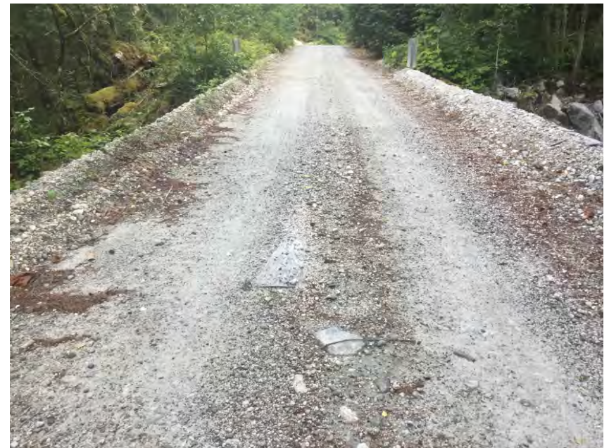
Exposed Stringer at Left Abutment
