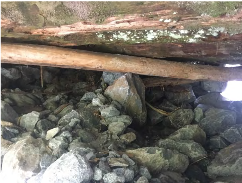
Debris Accumulation against Right Abutment
