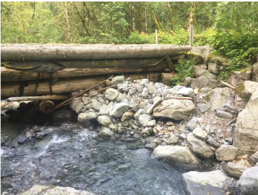
Accumulation of Rocks against Upstream Stringer
