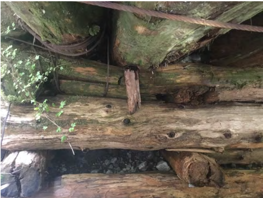
Left Abutment Collapsed Crib Log with Scour between Logs
